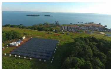
Impianto Off-Grid a Kitobo Island (2016)
