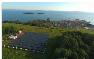
Impianto Off-Grid a Kitobo Island (2016)
